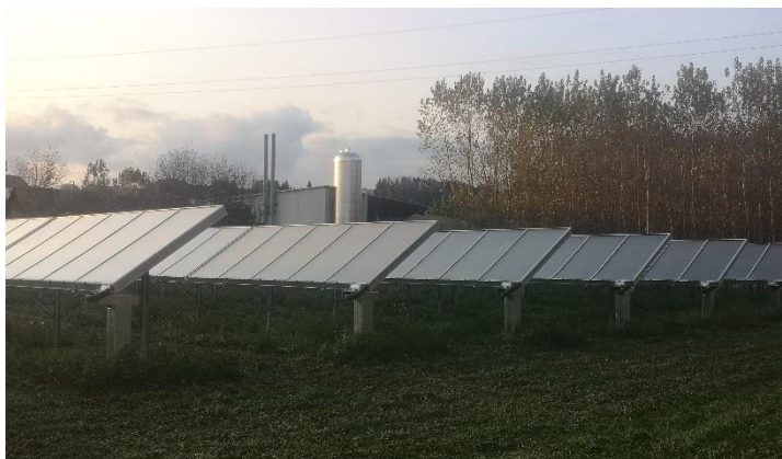
Freestanding solar thermal plants supporting the local distance heating (Austria).
